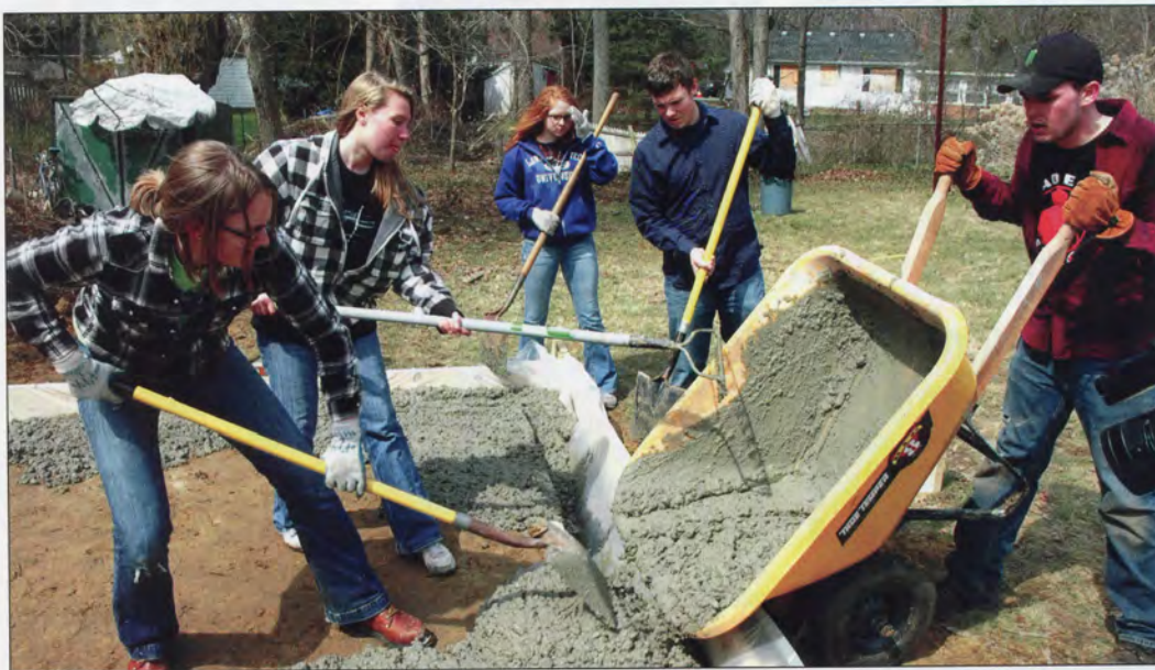
Pouring the concrete for a Freedom by Design project are (left to right) students Ellen Rotter, Samantha Doherty, Meaghan Markiewicz, Kevin Brown, and Michael Neal.
