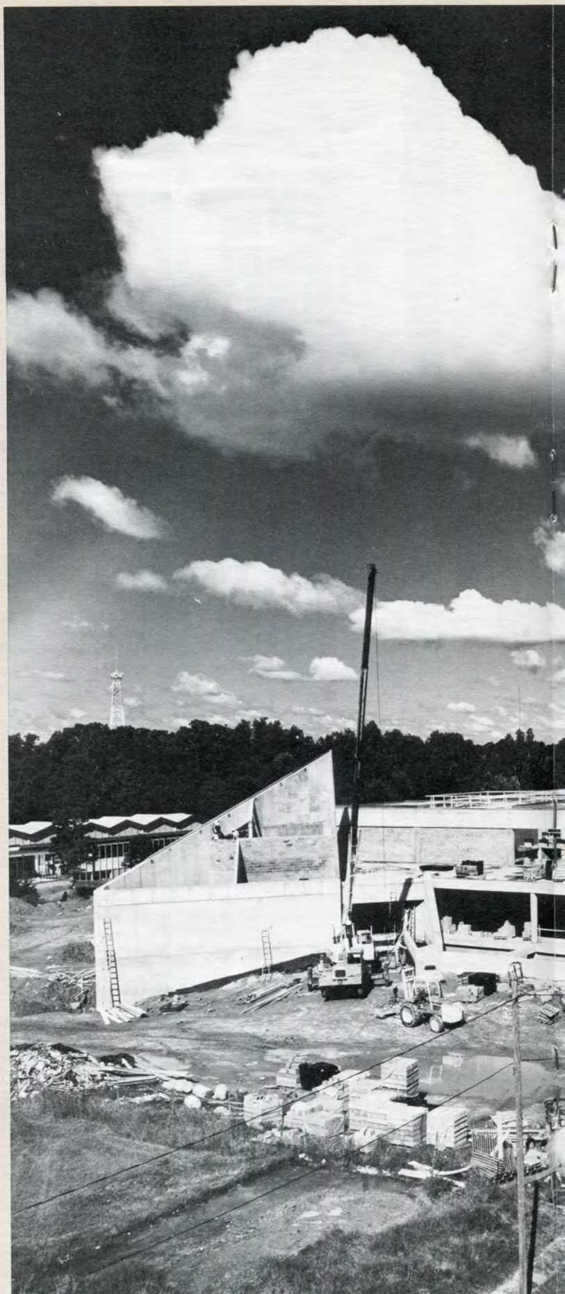
The new Management Building takes shape under the warm June, 1981 sun. The Building will also serve as library and dining facilities serving all students.
