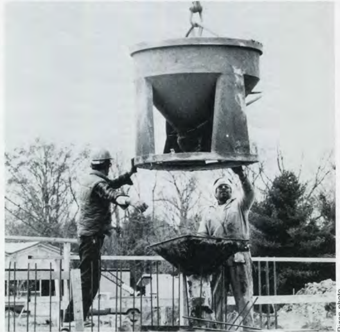
Underway The new Management Building will add approx. 100,000 square feet of badly needed academic space to campus.
