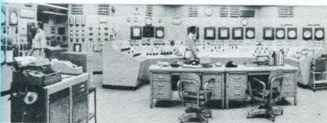
Enrico Fermi central control room where operators control plant manually or supervise operation of automatic systems. PRDC consoles and panels (left and center)-Detroit Edison equipment at right.
