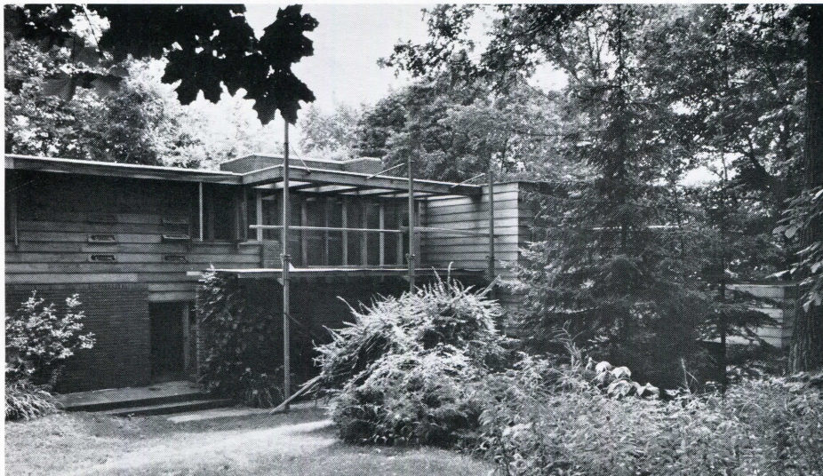
Scaffolding erected at LIT's Frank Lloyd Wright-designed Affleck House allows restoration of the home's cypress paneling and roof. Funding is being sought to restore the circa 1941 structure.
