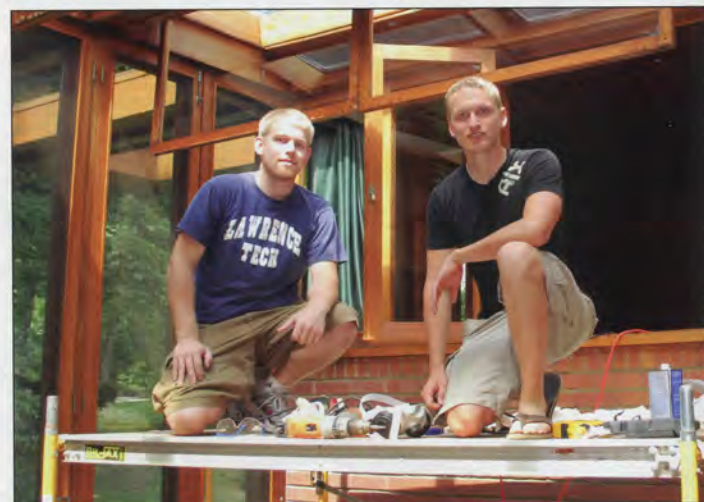
Lawrence Tech students Doug Metiva and Justin Butler have a good view of architectural history from scaffolding at the Affleck House designed by Frank Lloyd Wright.
