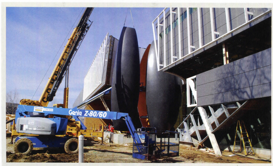
Shown during assembly earlier this year, a signature feature of the Taubman Complex is the spherical stairwell dubbed the "orb." It is one of the first structures built with fiber-reinforced polymer composites. More about the new building will appear in the next issue of this magazine.
