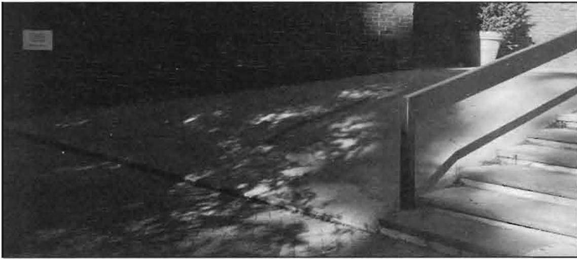
The ramp to the Union patio is too steep to be ADA approved.
