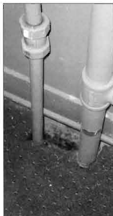
Pipes run through a hole in the floor of Room 23A. Although covered by carpet, the hole extends about 6 inches into the room.
