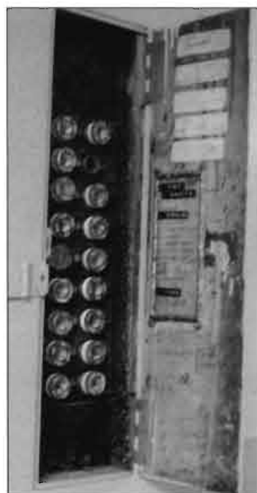
This fuse box, in the basement, like many others in the building, is not locked and accessible to anyone.
