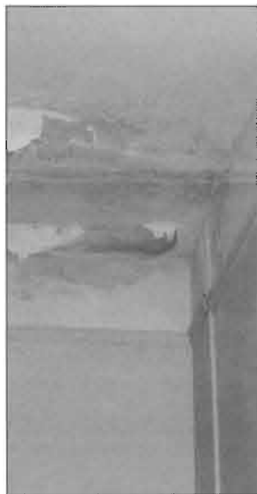
Room 22 has large sections of the ceiling peeling off in the back corner of the room.
