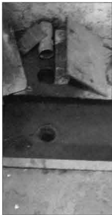
There is an open draining sink in the basement with standing water in it.
