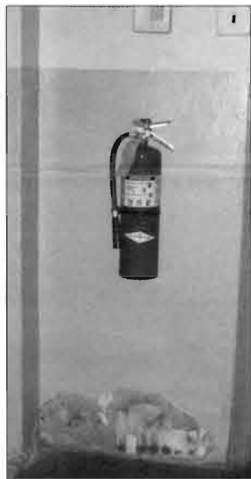
The wall next to B7 is worn through so the bricks behind it are beginning to show.
