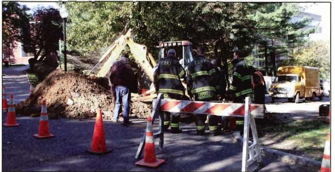
Construction crews digging behind the Union blocked off vehicular traffic onto campus for the entire day and night of Nov. 7.
