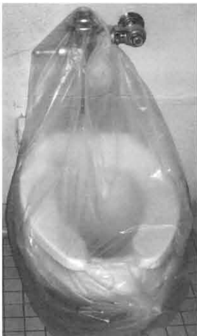
One of the unusable toilets
