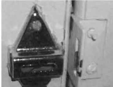
A missing lock from a bathroom stall
