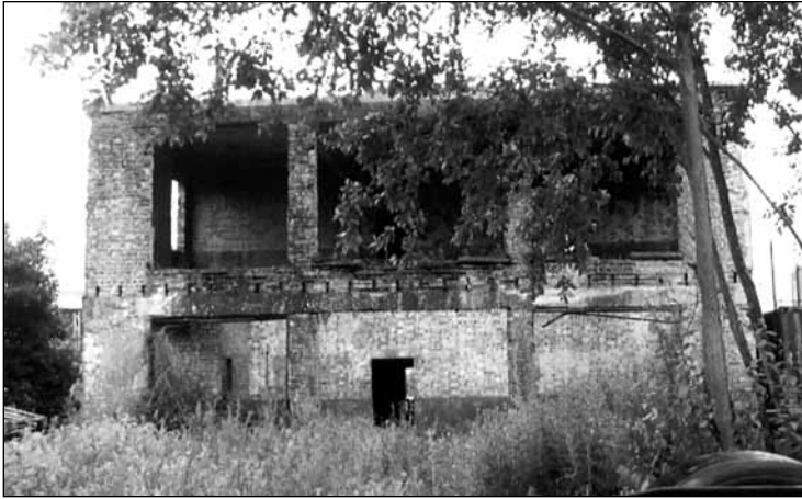
June 23, 2007: Mother Nature will gradually take over the Control Tower if restoration is never resumed.
