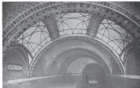
CITY HALL STATION OF THE NEW YORK SUBWAY, SHOWING GUASTAVINO CONSTRUCTION. Heins & La Farge, Architects.
