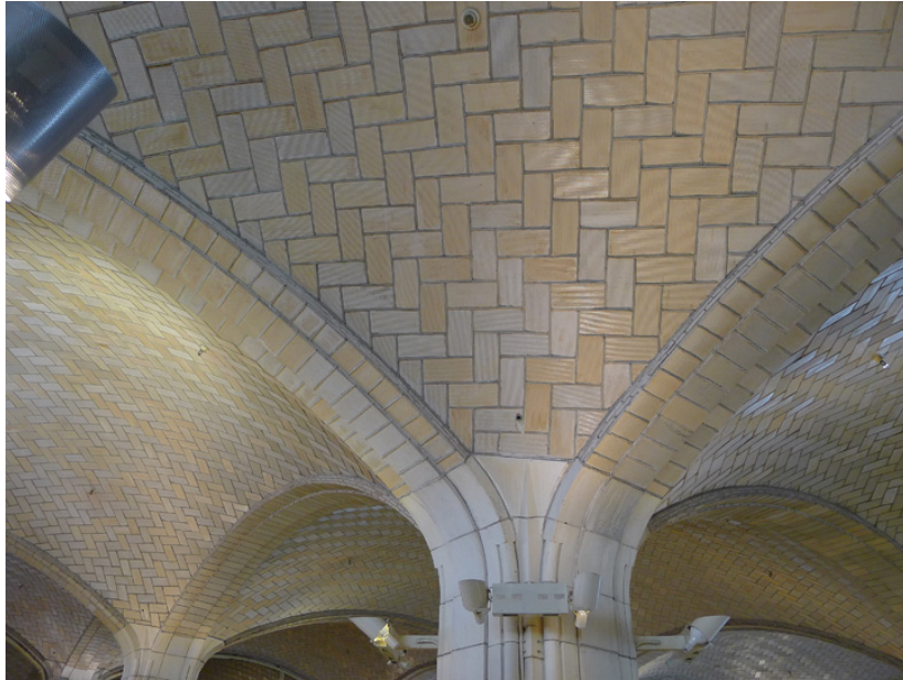
The Guastavino Company's tiled vaults under the Queensboro Bridge. (Photo courtesy of Michael Padwee)
