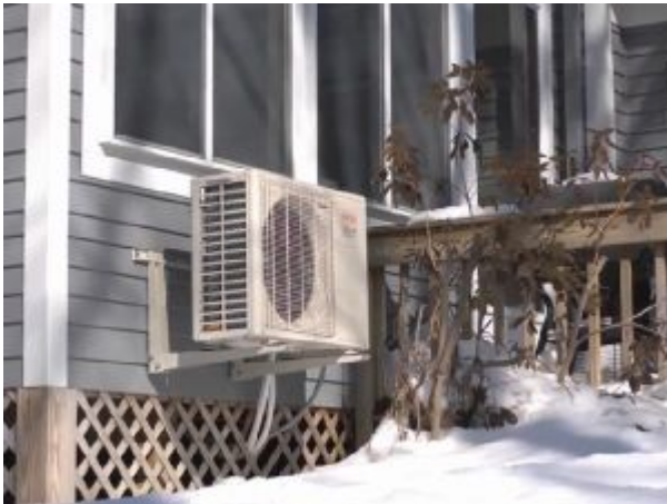
Since 2019, 40,000 heat pumps have been installed in Maine.
