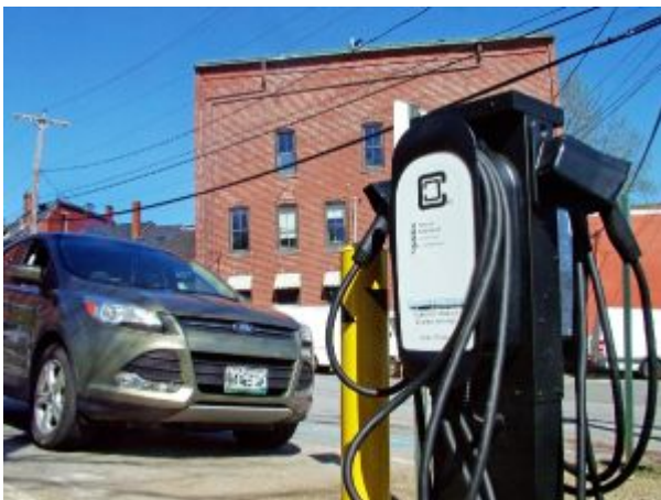
Electric vehicle charging station in Belfast. Photo courtesy Republican Journal.
