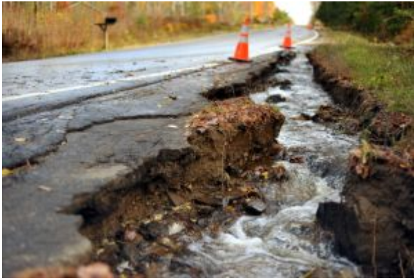
October 31, 2021 stormwater erosion on Poors Mills Road, Belfast. Photo credit: Fred Bowers.
