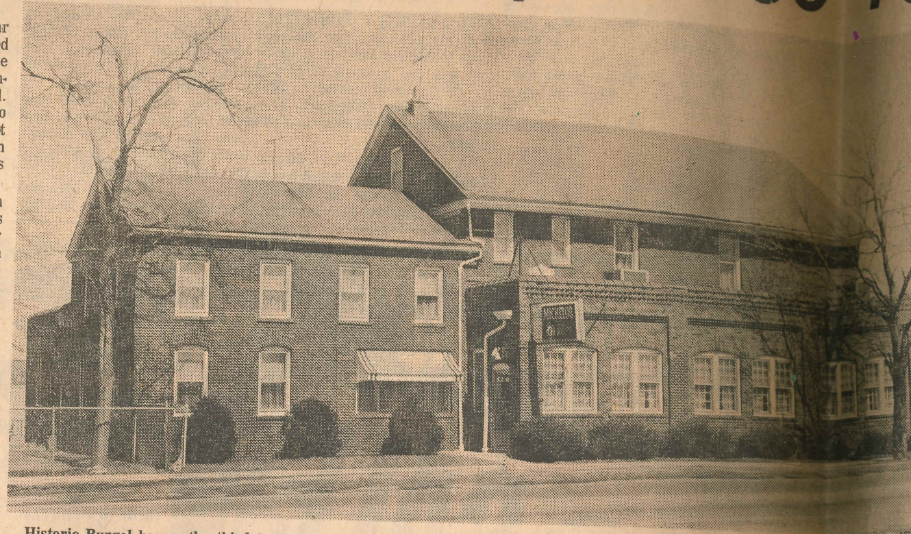
Historic Burgel house, the third tavern to stand on the northwest corner of Chicago road and Sauk trail, South Chicago Heights, is being torn down to be replaced by a contemporary ranch style Sinclair gasoline service station. The two-story red
