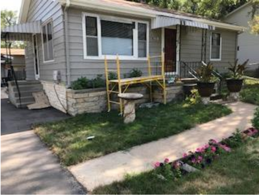
Painting in process. The outside color is called "elephant ear." In certain lights, it looks tan.
