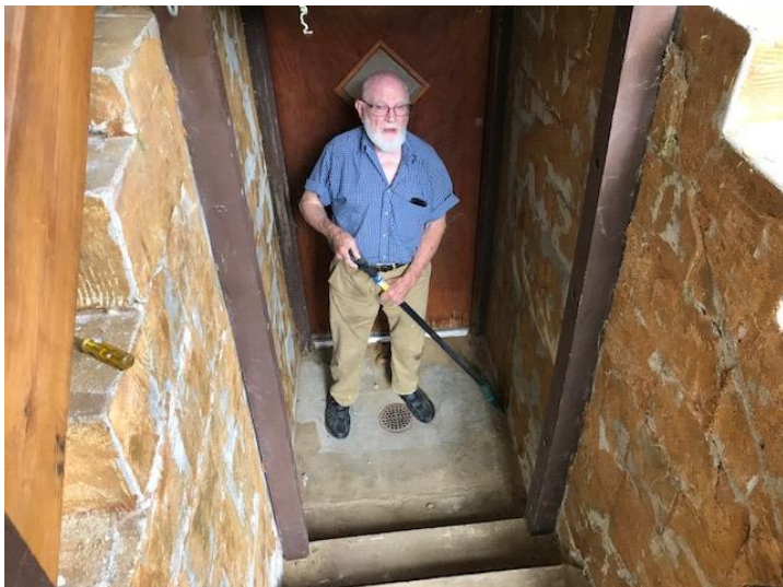
Dan after scraping green shag rug off stairs to basement, but before putting stucco on the walls.
