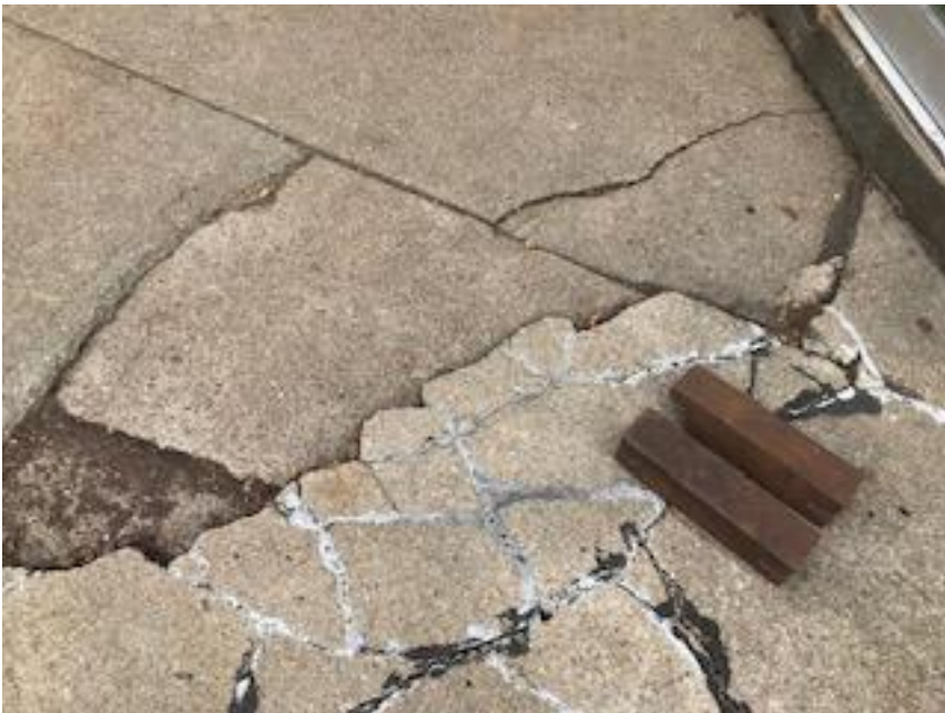
Close up of water damage on the driveway.
