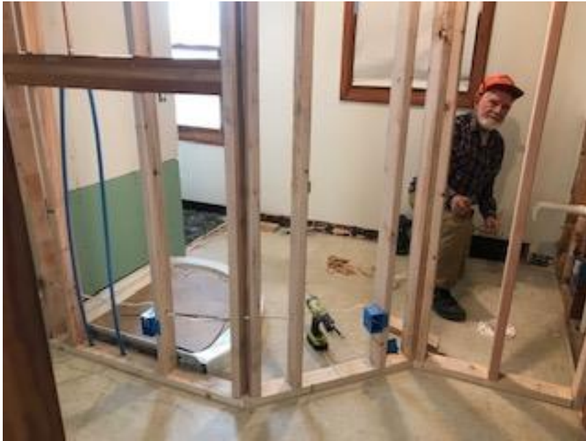
Dan designed and built the frame for the new bathroom but had the drywall and plumbing professionally done.
