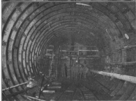
TUBE, before lining with concrete, each rib weighs 25,000 tons and is made of 2,400 cast-iron and 32 cast-steel rings, each 30 in. wide, 20, 204 segments held together by 210,769 bolts. AIR-LOCK, normal rib bulkhead wall, 10 ft. thick, three locks into pneumatic section.
