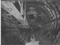
JUNCTION OF SOUTH TUBES , building last rings, Nov. 14, '06; bars made by driving 12 1/2-in. steel shield with 14 hydraulic rams exerting forward pressure of 4,000,000 lbs. Weight of shield and machinery, 197 tons. EMERGENCY AIR-LOCK for refuge in case of flooding.
