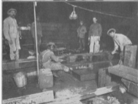
LINING AND WATERPROOFING rock section under Manhattan after excavation. LAYING DUCTS for electric power and light wires to carry the 100,000 electrical horsepower which will be required to move the trains and light stations and tunnels.
