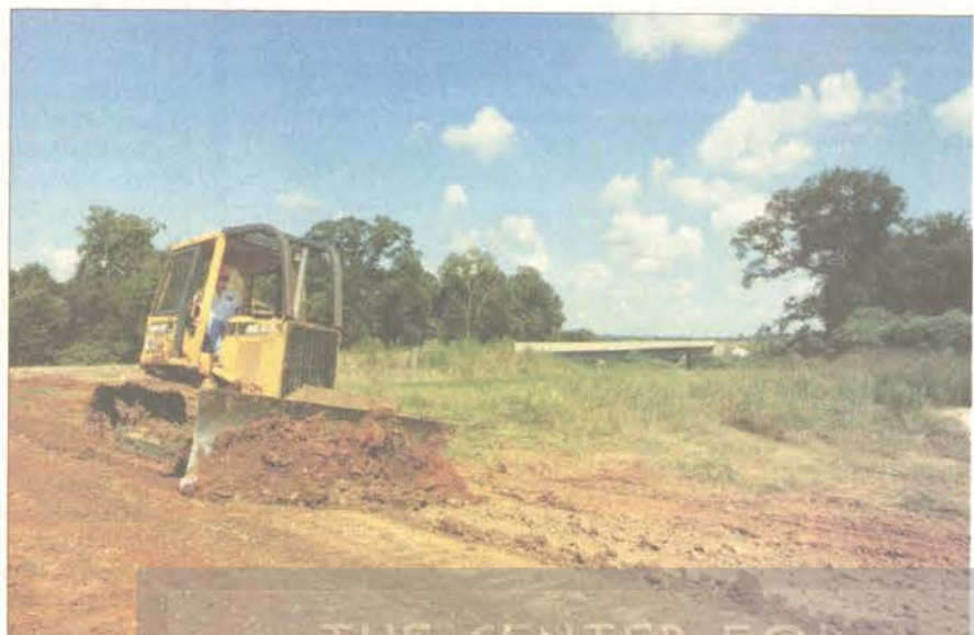
STAFF PHOTO | ROBERT SUTTON Mike Beard uses a bulldozer to prepare the road before paving starts on the Mitt Lary Road extension near the toll bridge on Black Warrior Parkway.
