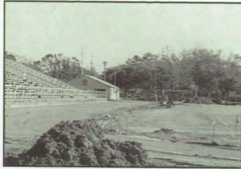
The messy dirt track of Bulldog Stadium is just a memory. A new track constructed of asphalt with a rubberized top is in the future of all running 'Dogs. photo by Renee Hamm
