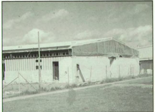
Construction of the foreign language building began in May of 1997. Many teachers and students were surprised to see that it was still not complete when they came back to school in August. photo by Roxanne Homuth
