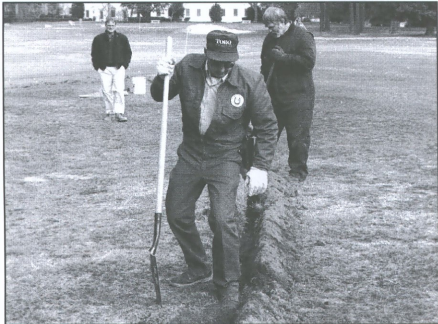
The maintenance crew at the Gold Course buries wire in the trench between the practice range and the first fairway. The wire connects sprinkler heads to an electronic box that automates irrigation along that portion of the course.
