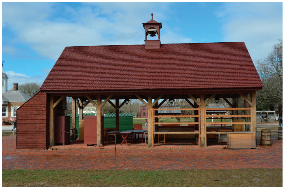
This February 2016 image of the Market House shows off its tar-painted roof.
