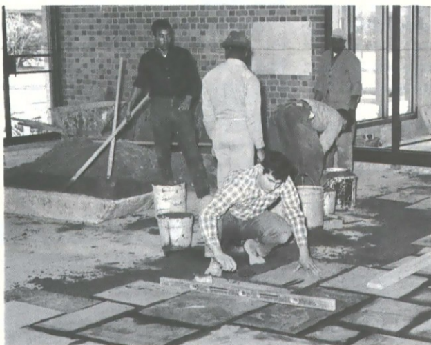
Above, workmen from Stonell, Stater and White Construction Company carefully lay the flagstone floor in the foyer of CW's new Cascades Restaurant in the Motor House area.
