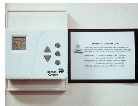
Thermostat levels are being customized to each area of the Foundation, with an explanation of the guidelines displayed in plain view.
