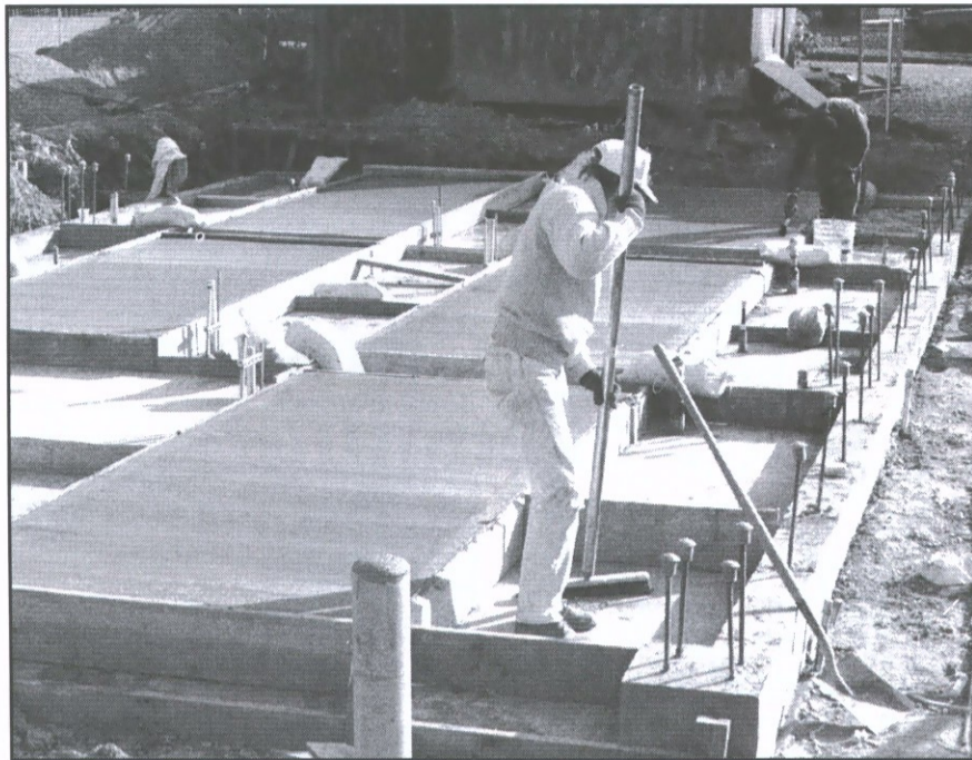
Subcontractors work on the concrete slab of the new natural gas fueling station under construction at the automotive shop. The slab was poured late last week. Construction of a concrete sound-baffling wall is the next step in the process. The refueling station is to be complete in a month or so.
