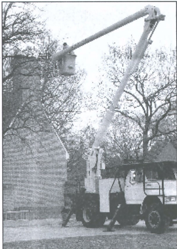
A cherry picker helps Colonial Williamsburg staff get the Governor's Palace ready for Grand Illumination. Christmas decorations and a sound system had to be put in place for the special event.
