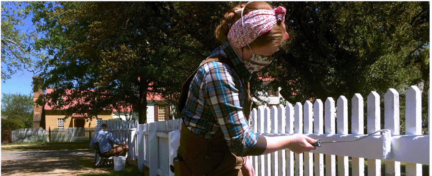
Aislinn Lewis, a journeyman blacksmith, paints a fence at the Roscow Cole House, following recommended COVID-19 safety precautions.
