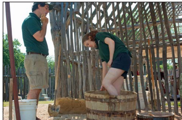
Colonial Williamsburg journeyman brickmason and supervisor Jason Whitehead and Emily Doherty make the mud to hold the walls on this building at Historic Jamestowne together.
