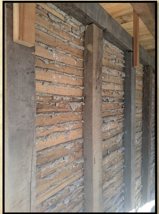
These are the keys that ensure the plaster is locked to the lath.
