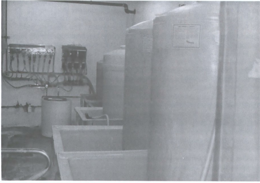
KEEPING IT CLEAN — New chemical storage racks with a computer-controlled dispensing system contributed to the Laundry's gold award from the Hampton Roads Sanitation District.
