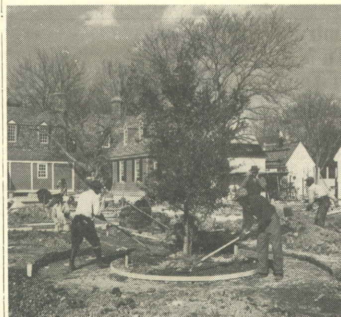
BEEHIVE of activity is the area behind King's Arms where finishing touches are being applied by members of the C & M Department.
