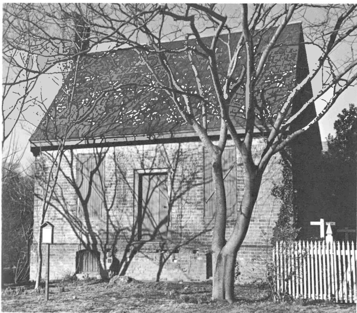
The eighteenth-century Greenhow-Repiton Office, traditionally known as the Debtor's Prison, before restoration.
