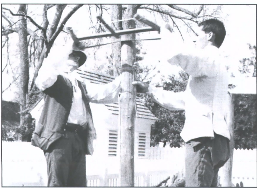
SHIELDS SHELTER — Historic Area carpenters begin work on a roof for the garden dining area at Shields Tavern.
