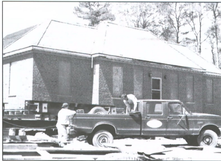
Workmen recently moved the home economics cottage at the Bruton Heights Educational Center 150 feet east of its former site.
