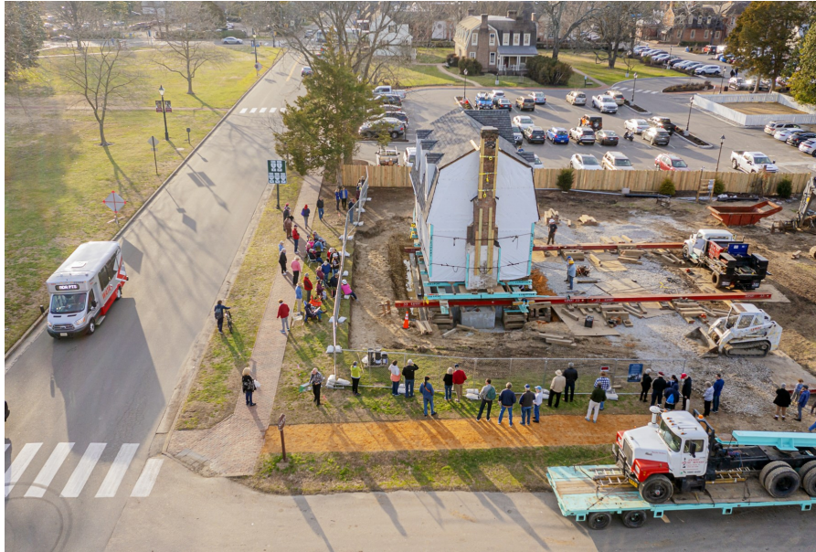
Aerial view of the Bray School atop its new foundation at Colonial Williamsburg. Photo by Wayne Reynolds.
