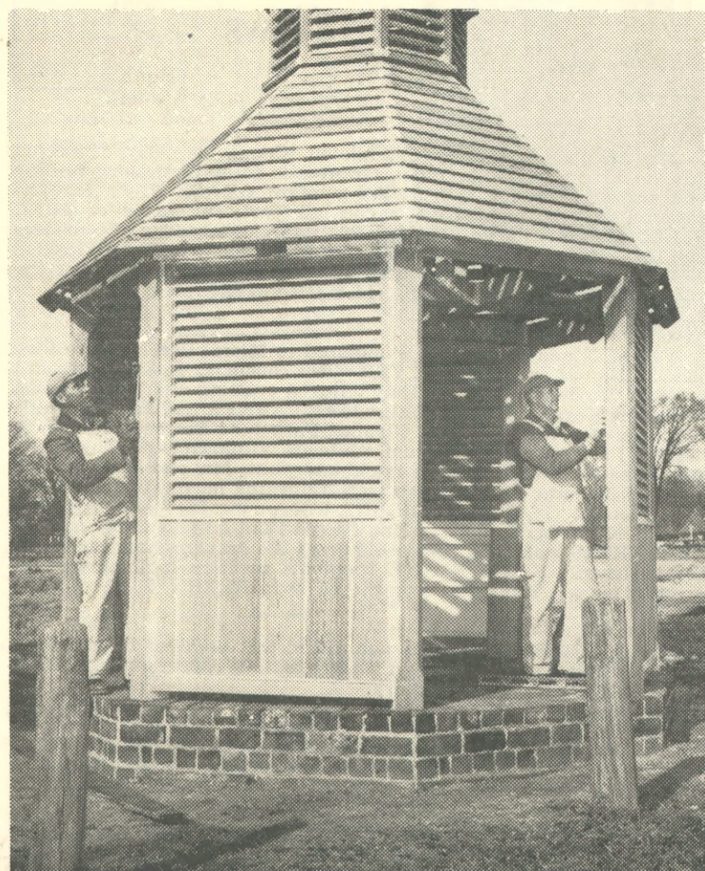
TOWN PUMP on Market Square Green begins to take shape as carpenters Charlie Perdue (left) and James Faris lend their skill to the task.
