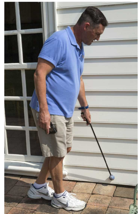
Using a tool he created, Joel Voron taps the wall near the foundation of the Bassett Hall teahouse, listening for the hollow sound that would alert him to possible termite damage.
