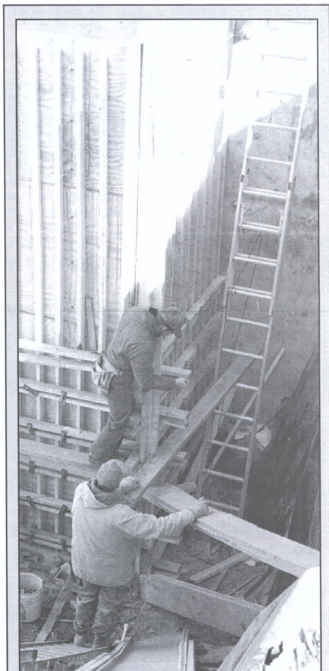
A VERY DEEP HOLE: Workmen remove forms used to pour an elevator shaft at the Cascades Restaurant and Conference Center. It's one of several improvements designed to make both floors accessible to the handicapped. Construction required a hole 20 feet below ground level. The project will bring the facility into compliance with the Americans with Disabilities Act. Photo by Jim Bradley
