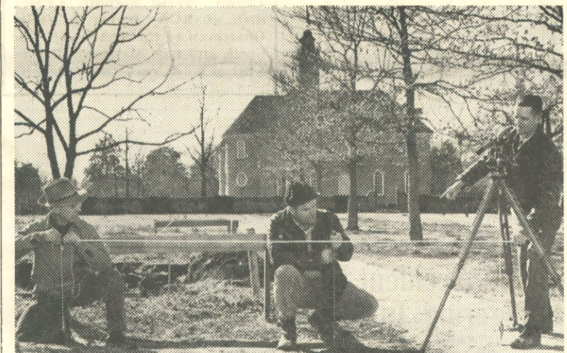
SURVEYORS (l. to r.) Charlie Thompson, "Shine" Moore, and Randy Carter with the equipment they use to determine locations of buildings and give grades to excavation and landscape crews.
