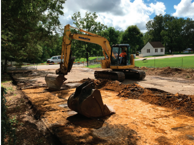
A contractor removes the asphalt parking lot that has covered the site of First Baptist Church since the 1960s.
