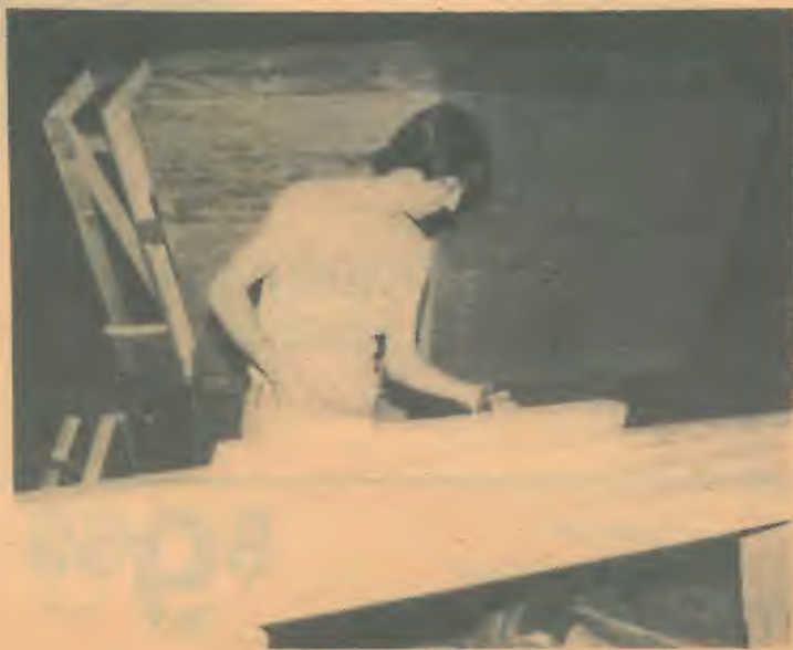
DISCO STATION - Workmen are making several changes to the Parliament House's Power House Disco including the construction of a new control booth for the sound and lighting technicians. Plans also call for resurfacing the dance floor according to resorpsomen. Other improvements and renovations will be taking place over the next few months and are scheduled to include a new window wall looking out on the resort's enclosed patio. (NDPic/Wesley)
