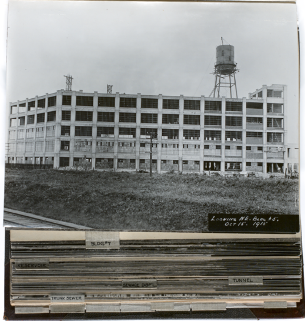
Canadian Kodak Co. [Looking north-east, building 5], October 15, 1915 Gelatin silver print, page 55 of album Kodak Heights 24.1 x 19 cm
