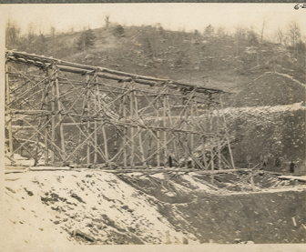
6-2 35 ft. Trestle across 173,000 cubic yard Fill Camp No 2 S & W R.R. This fill is 140 feet high on lower slope. Grade is 42 ft. above top of this Trestle 11/15/08
