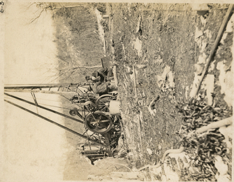
Drilling hole 83 feet deep on opposite cut. Well drill run with compressed air. 11-19-06
