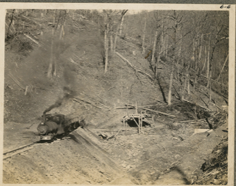
Putting in base of Fill 100 ft high over 8 ft Span Concrete Arch from above Shovel. 11-16-06
