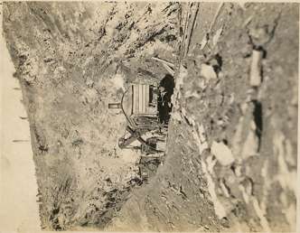
Shovel No 8 Camp No 2 S. & W. RR. working in 54000 cubic yard cut Station 418. 11.16-06
