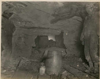
Where headings met in Lower Bridle Path Tunnel Camp 3 S.E. W. RR. Allapass N.C. 10-1-07.
