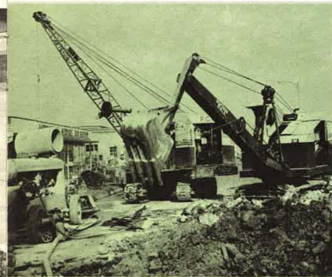
A temporary inconvenience while more sanitary and storm sewers are installed to serve you better.
