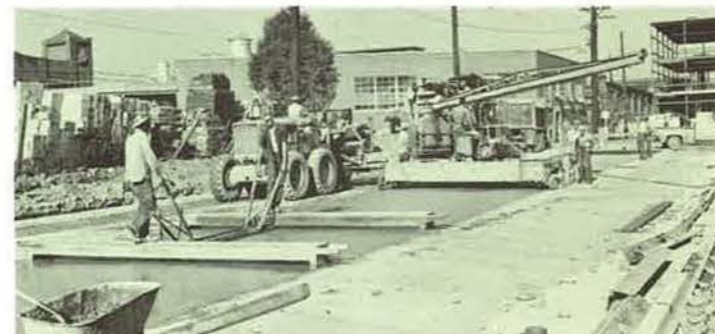
10,118 cubic yards of concrete used in paving and repairing streets and sidewalks in 1960-61.
