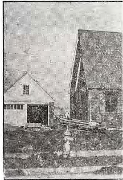
This new home, now rapidly nearing completion. Every little detail has been carefully studied. Huddle and is located on Lyaville street in Kingsport.
