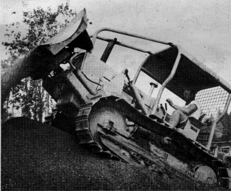
Construction activity on the Green River campus is in full swing as workers battle to meet at January deadline on some of the buildings.
