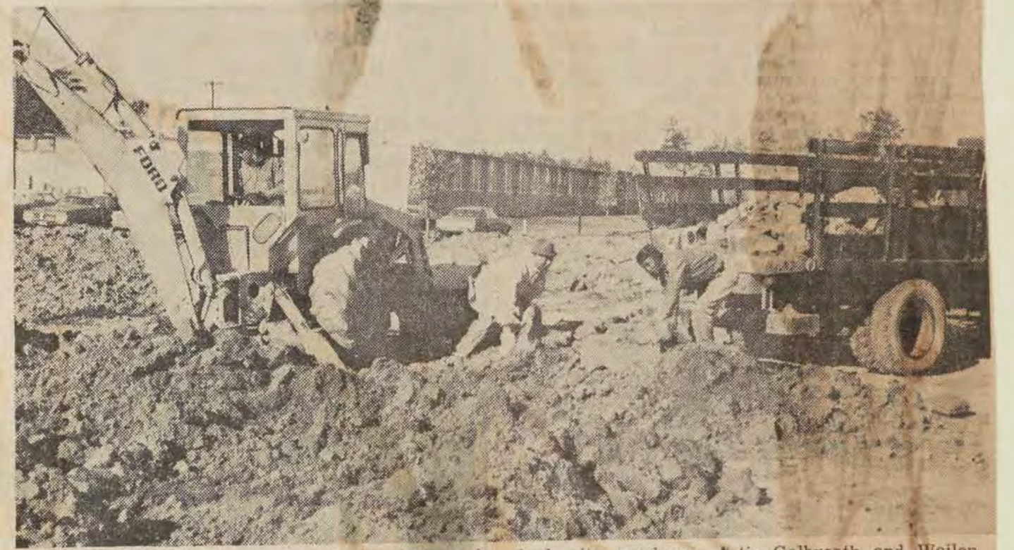
GARDEN SITE — Workmen clear the foundations of the old Honeycutt housing units in preparation for the City Rose Garden at the corner of Hull Rd. and Devers St. Shown are (left to right) Andrew Saut-
