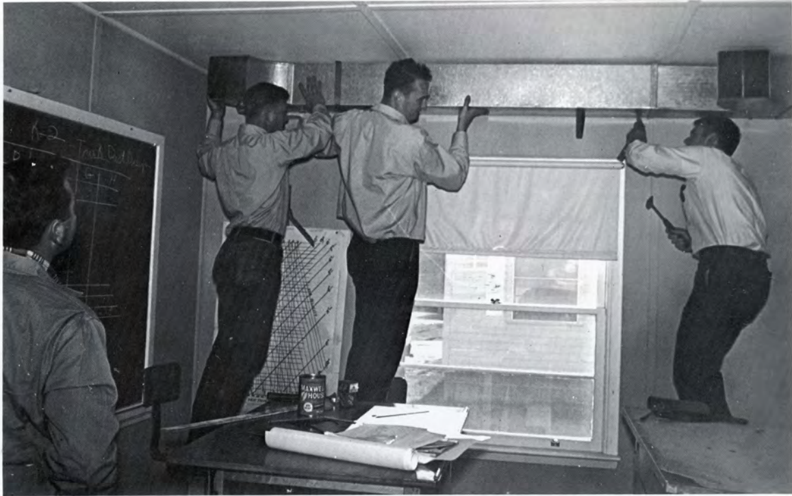
Practical application of fabrication and installation of duct work is performed by the students in the above picture.
