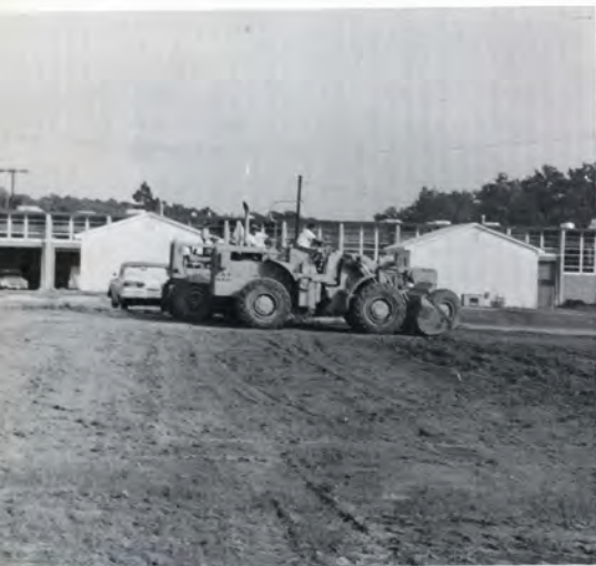
Heavy construction equipment cleared the area for the new parking lot and building site.
