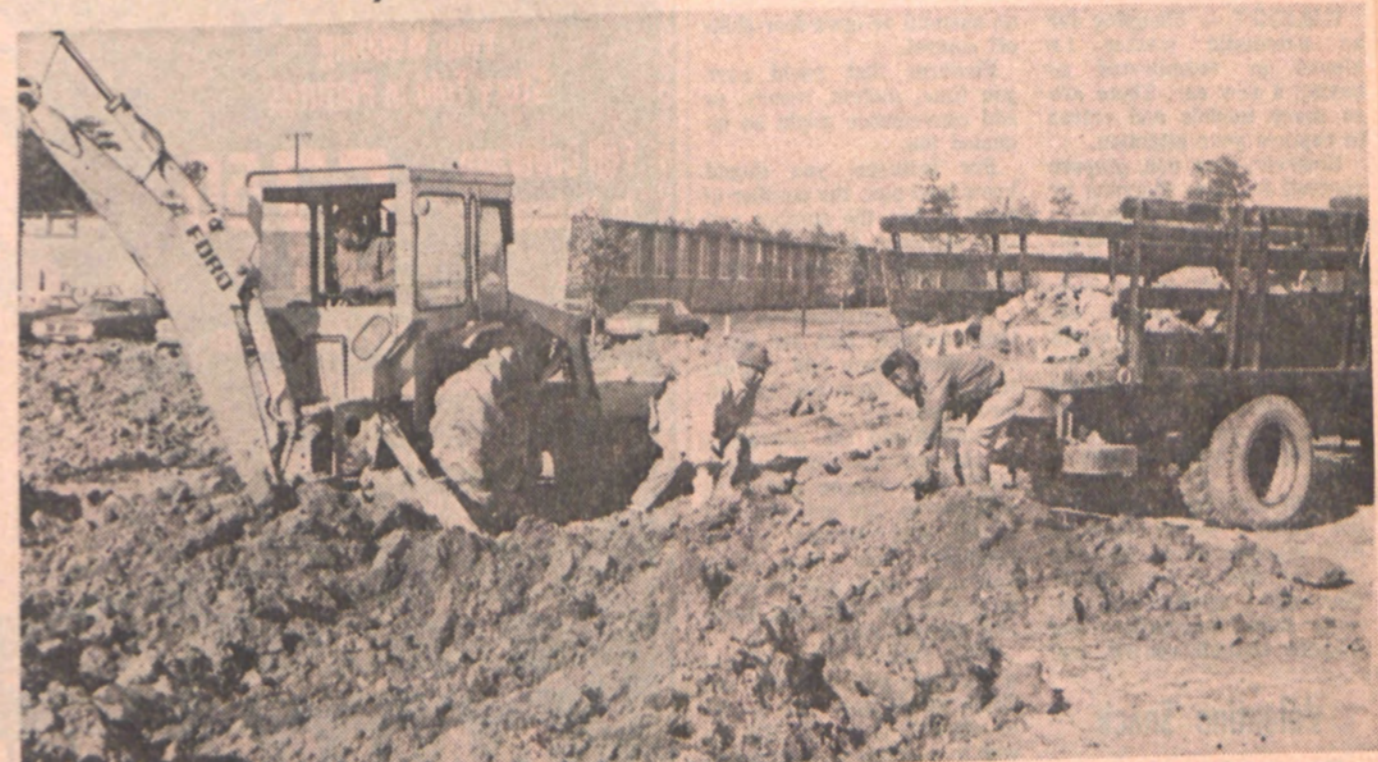
GARDEN SITE — Workmen clear the foundations of the old Honeycutt housing units in preparation for the City Rose Garden at the Corner of Hull Rd. and Devers St. Shown are (left to right) Andrew San-
